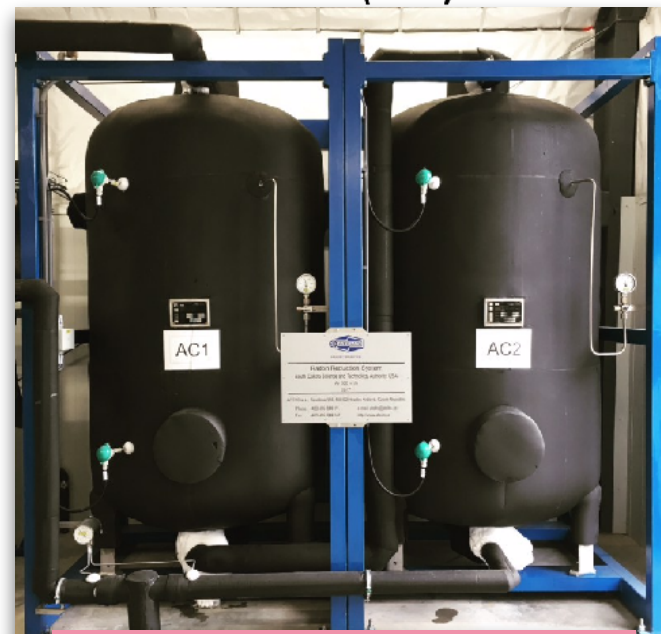
Radon reduction system at SURF
